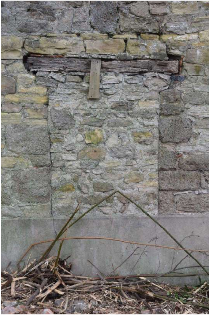
Photo 29 (left): Blocked doorway in the ground floor of the south face of the eastern extension, looking north
